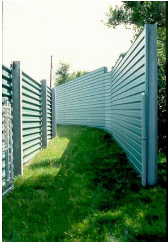
Figure 20. Example of overlapping barriers photo #5902
